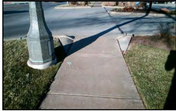
Corner 2 No Ramp (2z)
