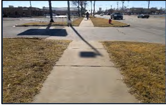
Corner 2 No Ramp (2z)
