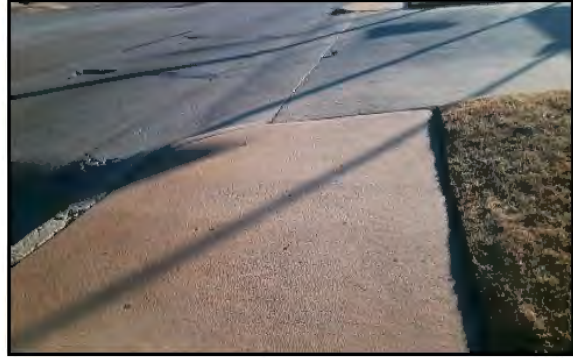
Corner 4 No Ramp (4z)
