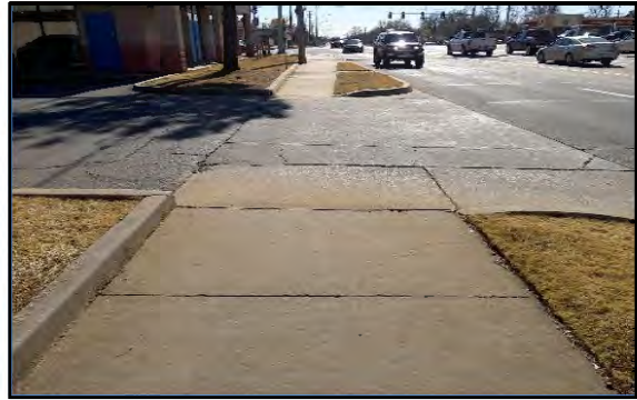
Corner 2 No Ramp (2z)
