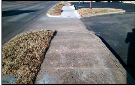
Corner 2 No Ramp (2z)
