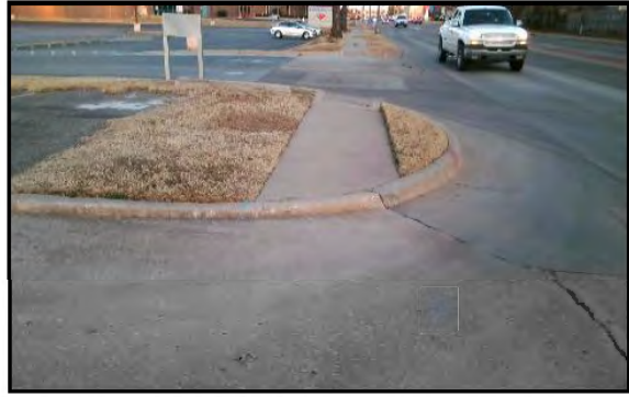
Corner 2 No Ramp (2z)
