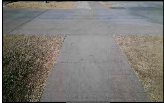
Corner 2 No Ramp (2z)
