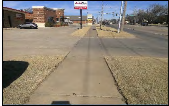
Corner 4 No Ramp (4z)
