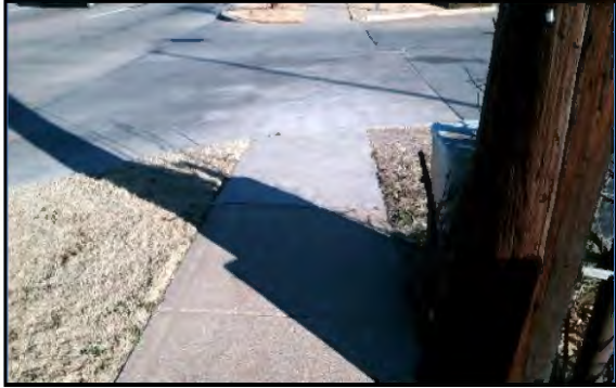
Corner 3 No Ramp (3z)
