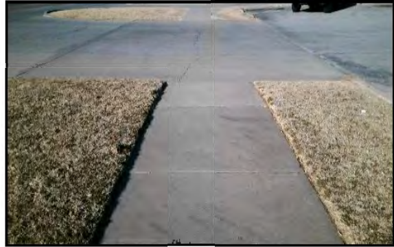
Corner 2 No Ramp (2z)
