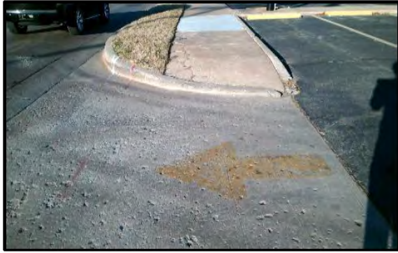
Corner 1 No Ramp (1z)
