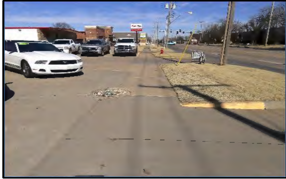
Corner 1 No Ramp (1z)
