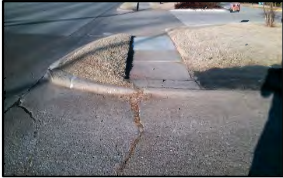
Corner 1 No Ramp (1z)
