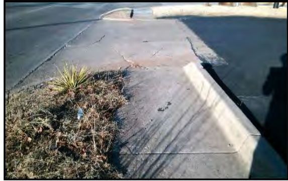
Corner 2 No Ramp (2z)
