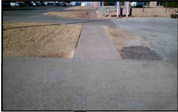
Corner 1 No Ramp (1z)
