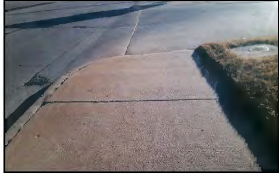
Corner 4 No Ramp (4z)
