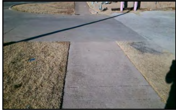
Corner 2 No Ramp (2z)
