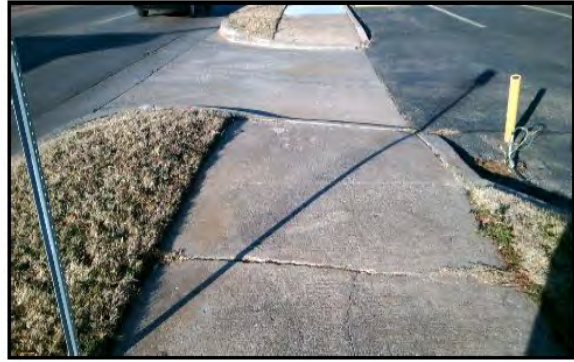
Corner 2 No Ramp (2z)
