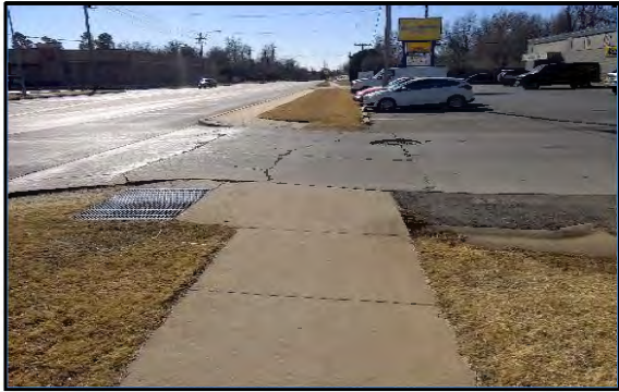
Corner 1 No Ramp (1z)
