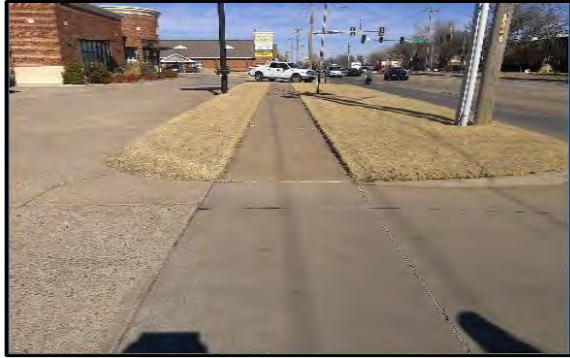
Corner 1 No Ramp (1z)
