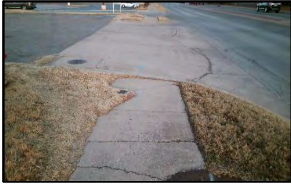
Corner 1 No Ramp (1z)
