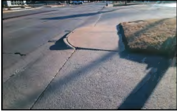
Corner 3 No Ramp (3z)
