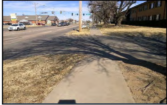
Corner 3 No Ramp (3z)
