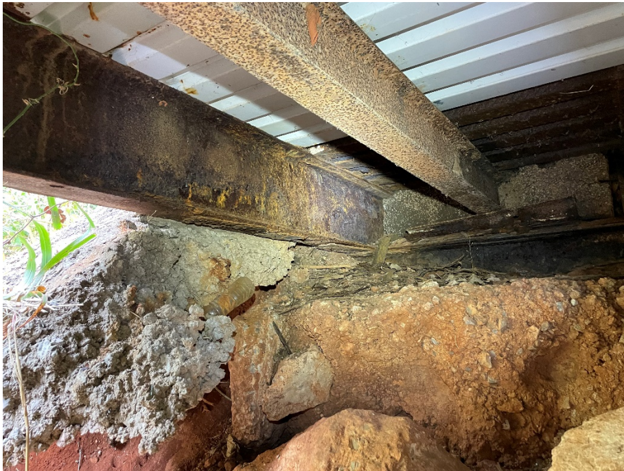
Loss of section to end of beam 1 at north abutment
