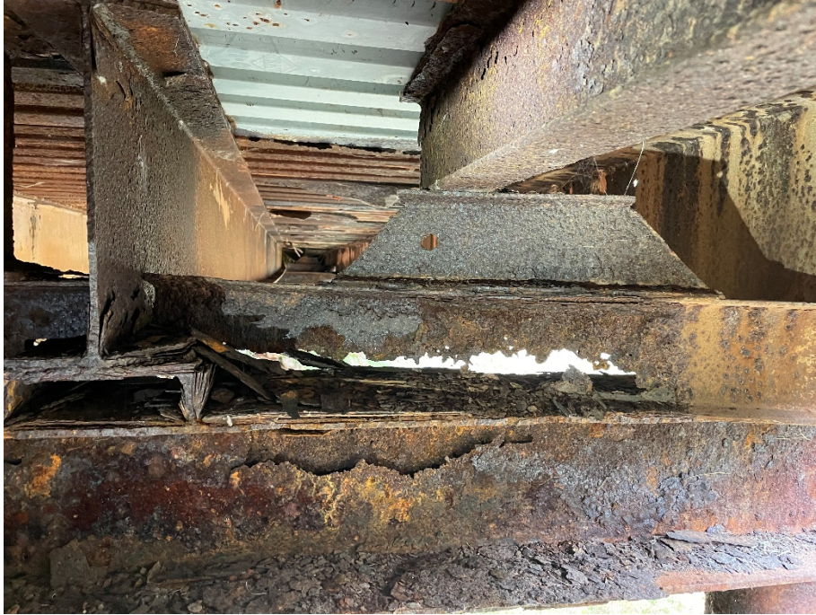
Section loss to secondary support on pier cap at east end
