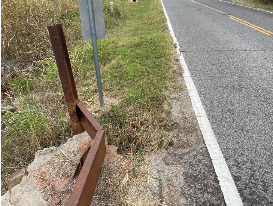
Southeast ditch erosion, looking south
