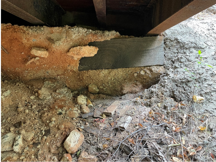
Erosion at west end of south abutment
