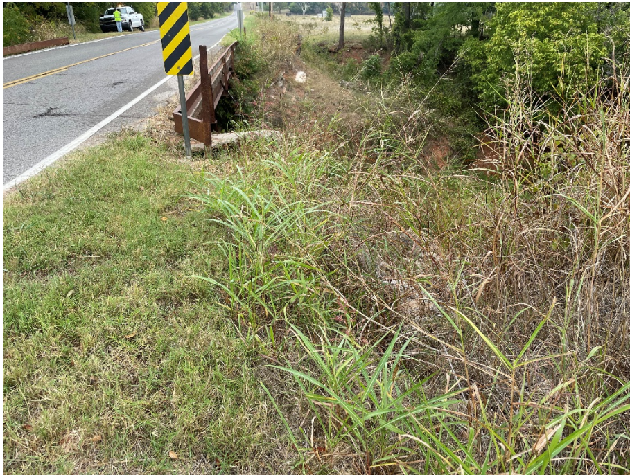
Southeast ditch erosion, looking north
