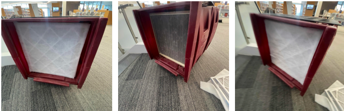
36. Third Floor - Main Area: Filter Change
