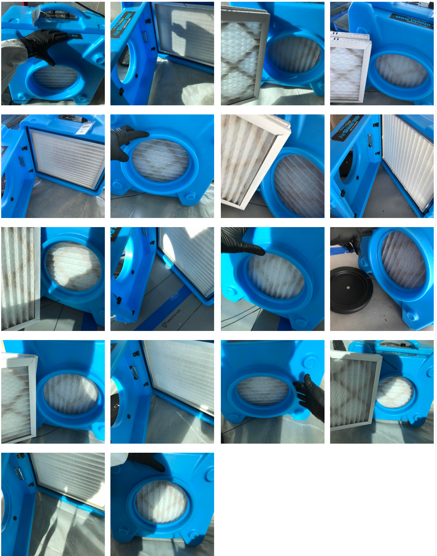
29. Second Floor - Main Area: Filter Change
