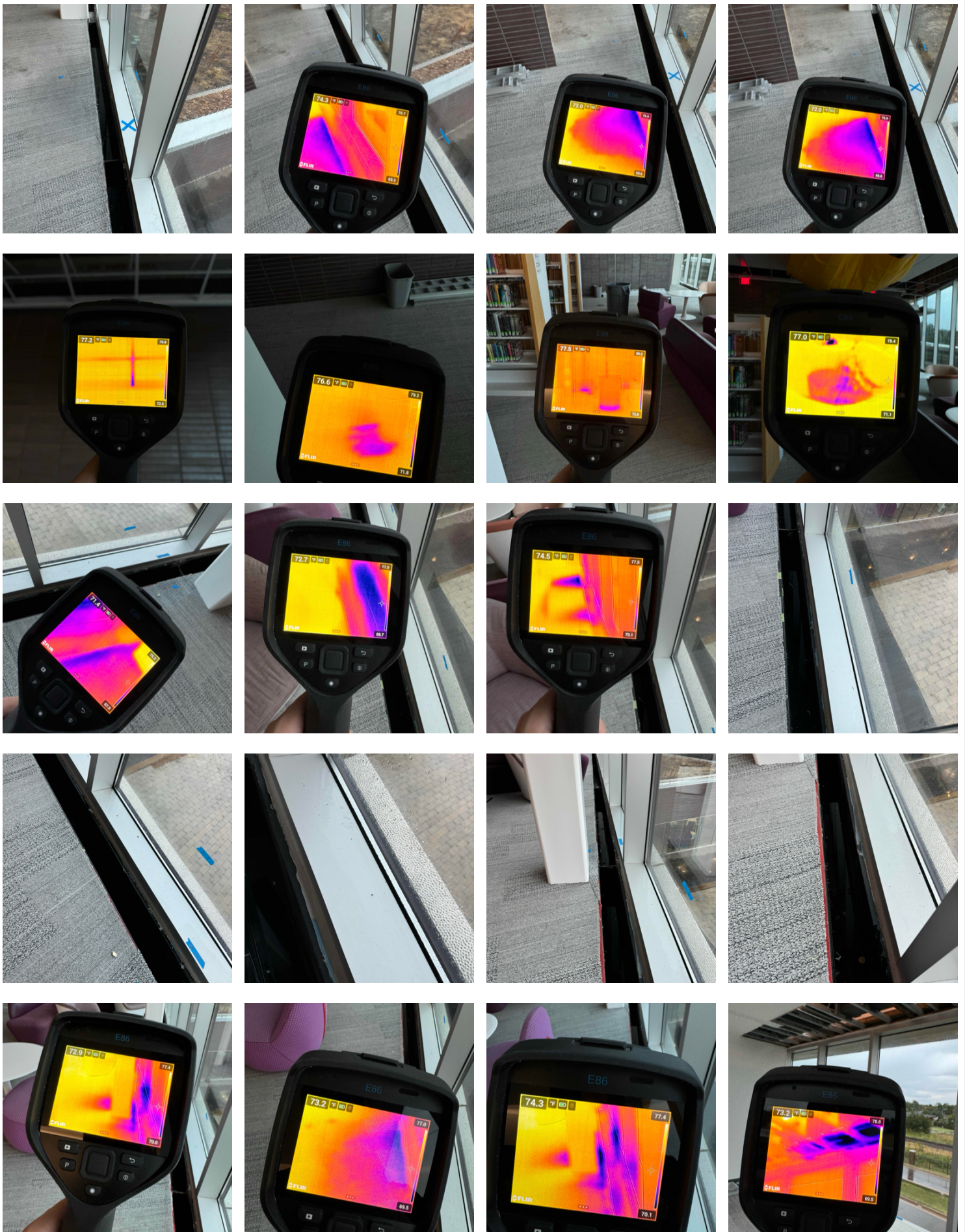
13. Study room-231: Thermal imaging and visual inspection show signs of residual water actively collecting inside the HVAC
