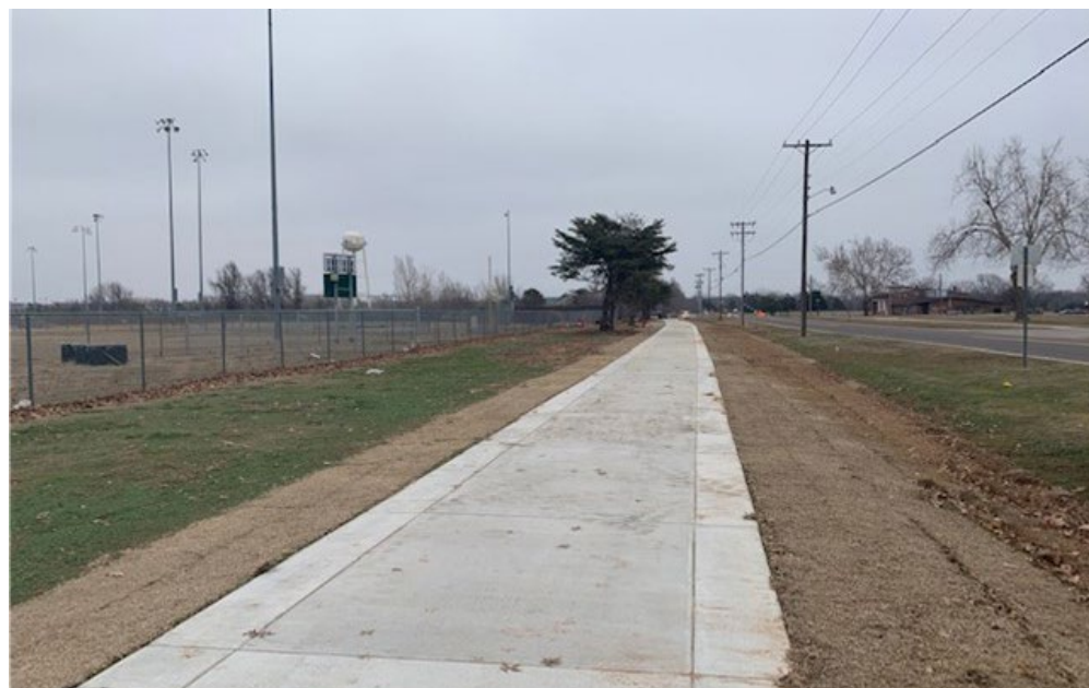
Completed Constitution Street Multimodal Path between Jenkins Avenue and Classen Boulevard North Side of Street
